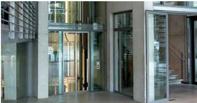
Lift fixings, guide rails
